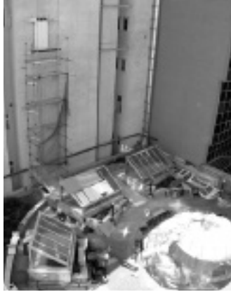
▲ A glass elevator, now under construction, will provide direct access to facilities at Zrínyi Street 14.
